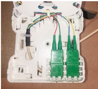
Special configuration in accordance with the specifications of the German subsidized fiber optic rollout
